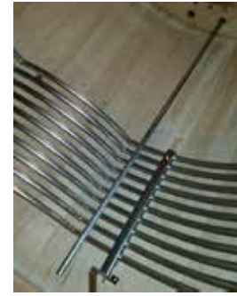
MLP sensors inside the tank.
